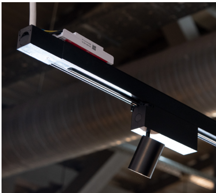
◀ Zumtobel installed 34 Supersystem II spotlights controlled via qualified Bluetooth mesh bmLINKs and a LITECOM controller
